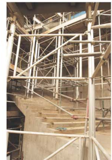
Existing scaffolding preventing construction of public stair.
