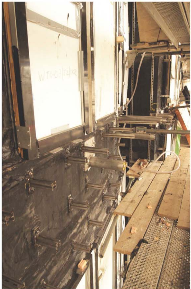
Blast Window Installation: problems with installation to meet blast proofing requirements mean that the installation rate has been cut from a projected 24 per week to 12 per week
