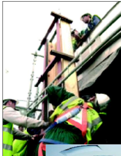
Drawn Metal staff lowering windows into place on one of the Committee Towers.
