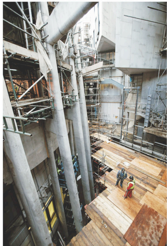
The installation of the high level crash deck in the North Lightwell.
