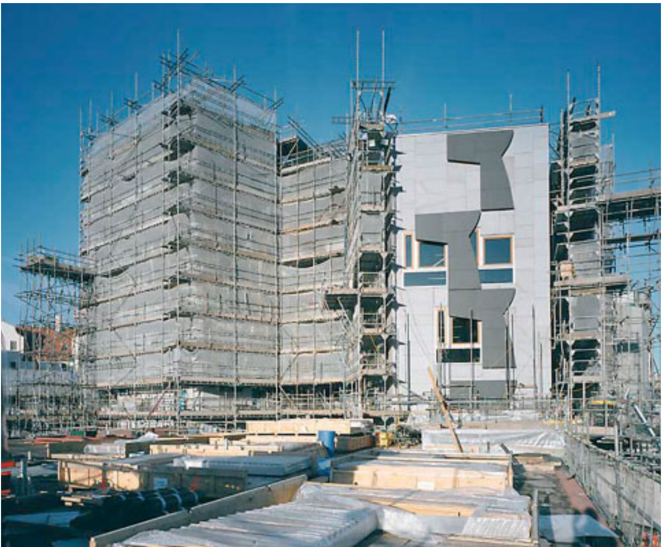
Trigger panels on Tower 1
